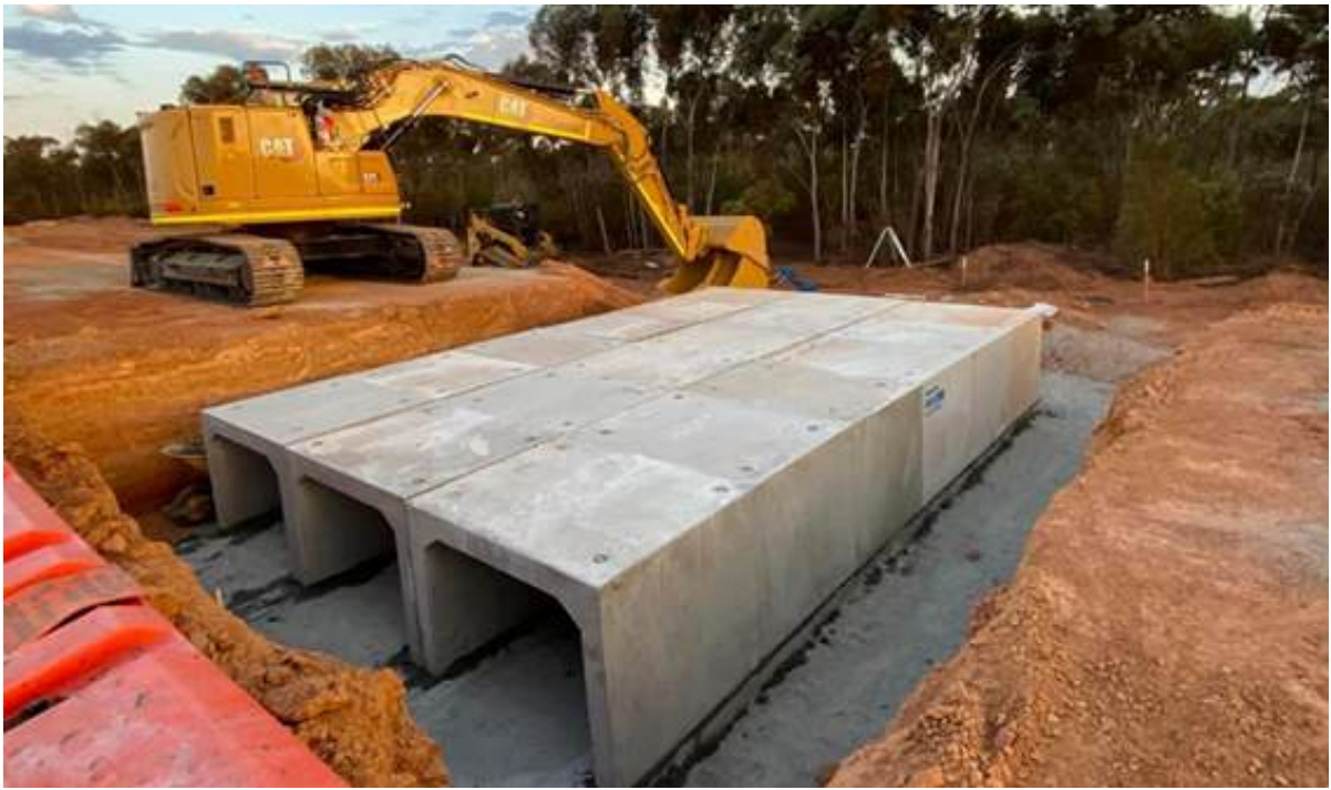
Above - Installation of base and crown units to one half. | Below - Aerial view of project.
